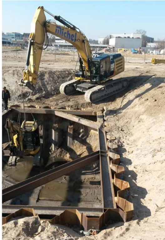
Preparing the ground: construction subsidiary omniCon cleaned up oil damage at Zollhafen Mainz
