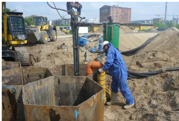
Preparing the ground: Site development by specialist construction subsidiary omniCon in Berlin's Europacity
