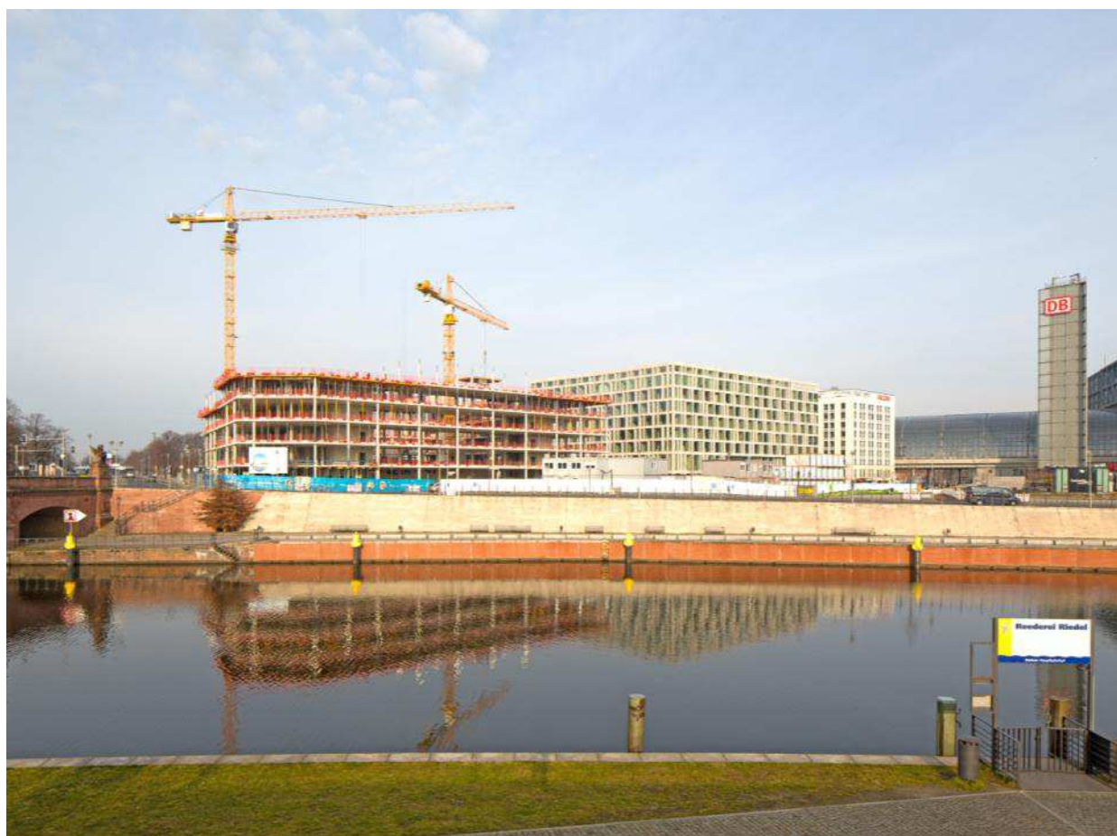
John F. Kennedy Haus construction site in the Berlin urban district Europacity
