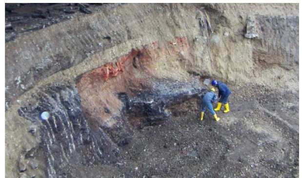
Preparing the ground: site development by specialist construction subsidiary omniCon in Munich's Arnulfpark
