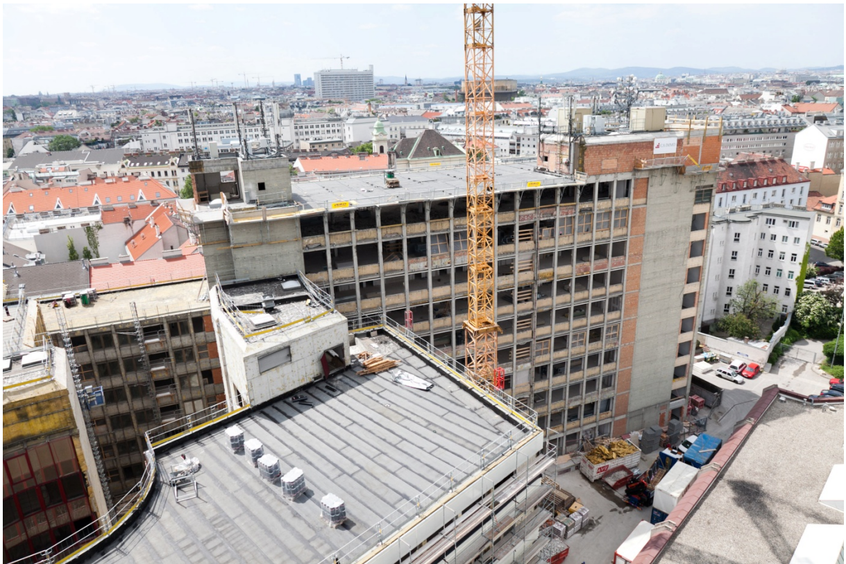
In May, CA Immo celebrated the topping out ceremony for the office building „Silbermöwe“ at the Vienna Lände 3 site
